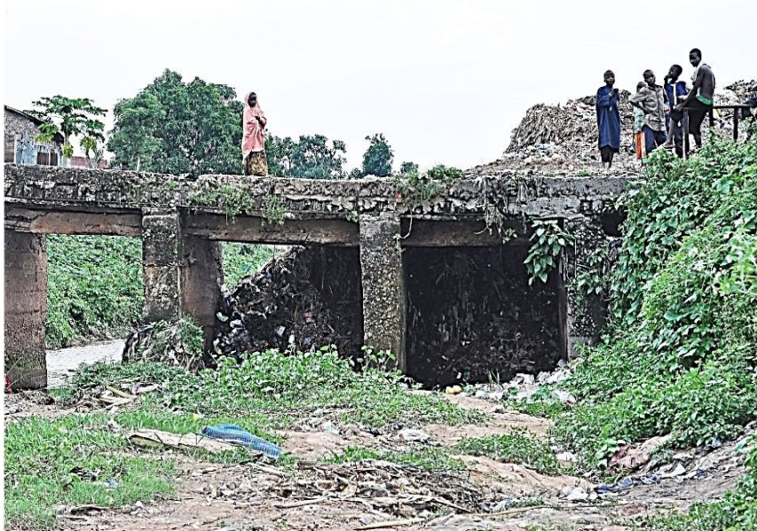
Figure 6: Another heap of Solid Waste Generated covered the bridge of Okpa Go-Os
