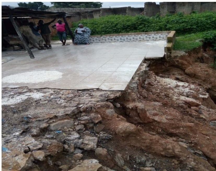
Plate 5: Soil erosion trespassing Garri processing plant near Angwan Nungu, Lafia North
