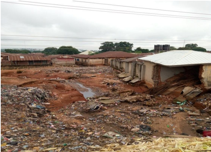
Plate 3: Soil erosion usurping houses along Makurdi road, Lafia Central
