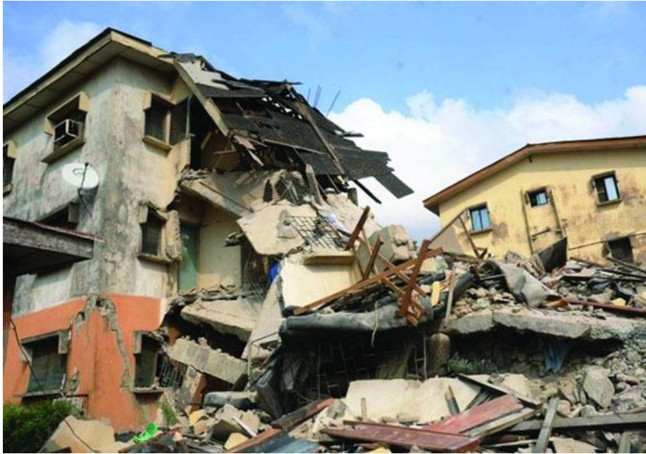
Plate 1: Location Gwarimpa State: Date March (2013) Source: National emergency management Agency 2021
